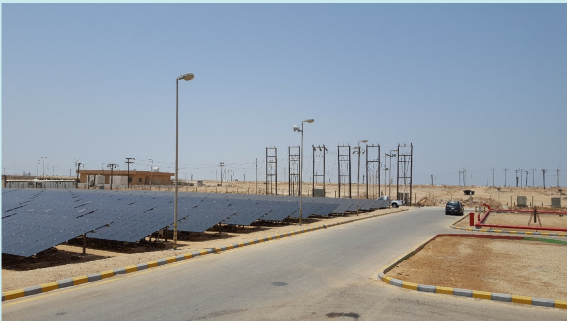
Figure 3. PV Solar Energy with RO has been implemented in since 2016 in Farasan Island, Saudi Arabia through the Solar Desalination project
